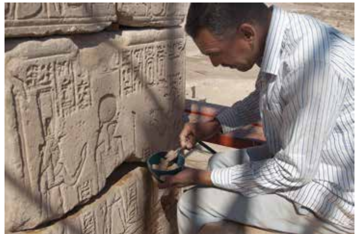
Saber working on the mortar of the Domitian Gate. Photo by Sue Lezon
