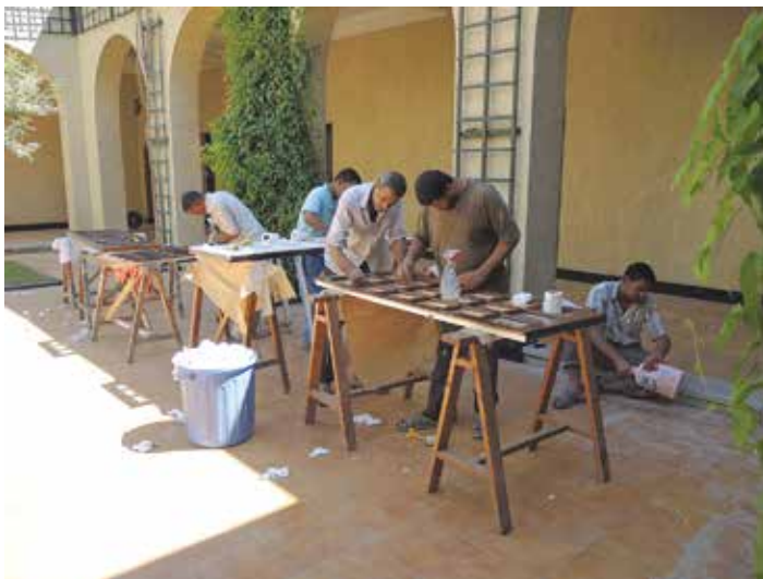
Sanding dining room windows. Chicago House. September 2014. Photo by Tina Di Cerbo
