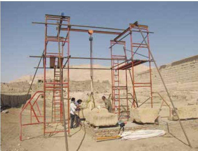
Roof-block restoration at Ramesses III well. Medinet Habu . December 2014. Photo by Nahed Samir
