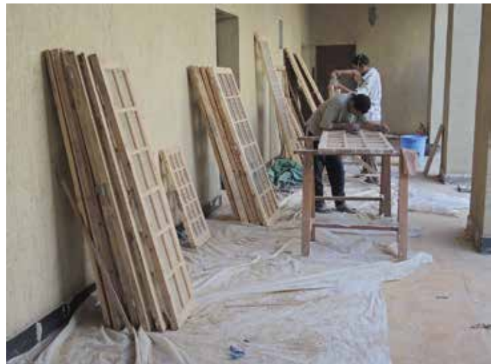
Staining and painting dining room windows. Chicago House. September 2014. Photo by Tina Di Cerbo
