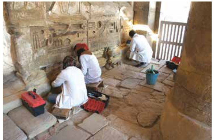
Conservation students consolidating decaying northern wall. Medinet Habu small Amun Temple. Photo by Ray Johnson
