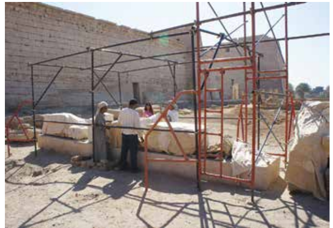
Southern well blocks being wrapped for the summer. Medinet Habu. April 2015. Photo by Ray Johnson
