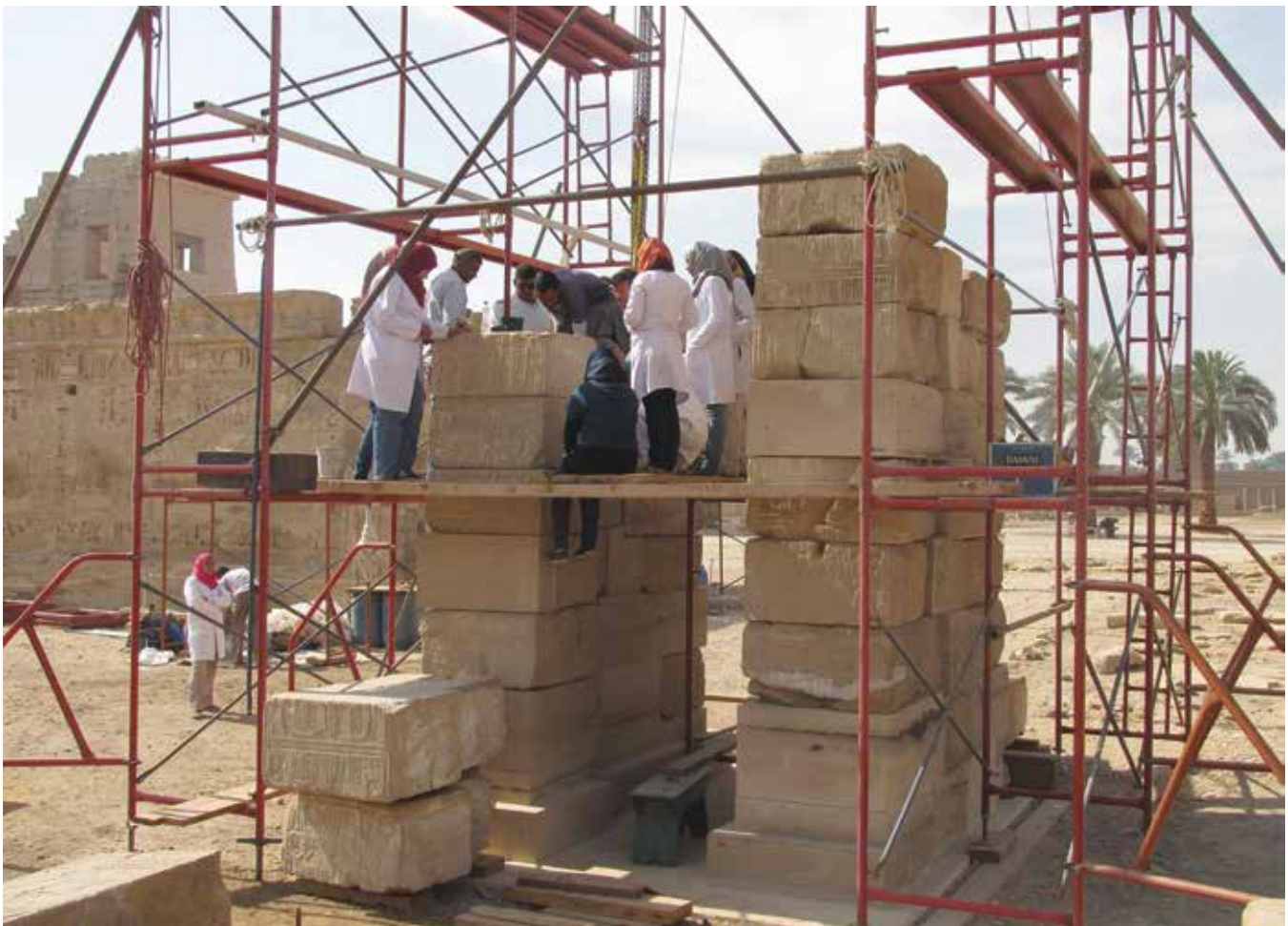
Conservation and restoration teams working together on the Domitian Gate. Medinet Habu. March 2015. Photo by Lotfi Hassan
